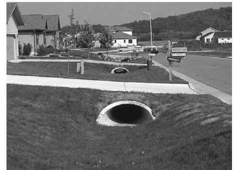
Swale replaces ditch.
