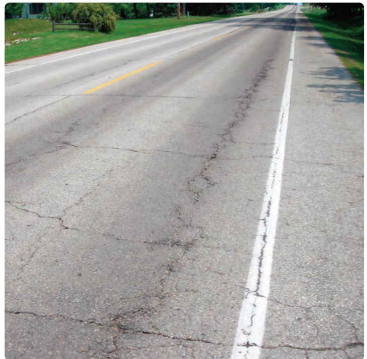
Rating this asphalt pavement a 4 on the PASER scale due to longitudinal cracking in the wheel path indicates the need for structural improvement with an overlay or full-depth reclamation. Choosing a maintenance or improvement approach that effectively extends the life of a road depends on an accurate condition rating.
