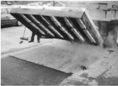
Infrared heater softens asphalt around a raised manhole, readying it for repair.
