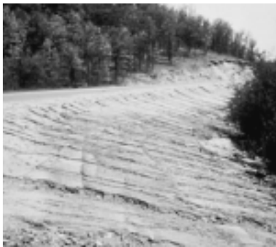
Protect exposed ditch soil from erosion. Seed immediately and use erosion control blankets.
