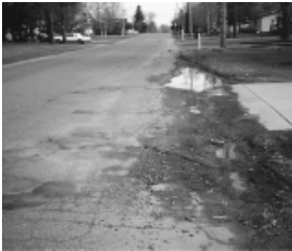
Roads with poor crown and no shoulder or ditch will suffer pavement failure.
