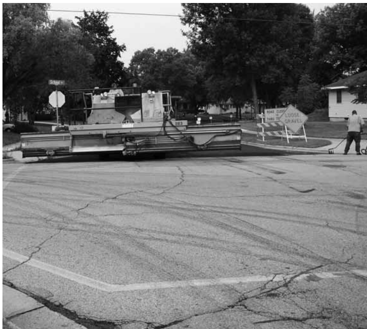
Pavements are ready for crack filling and chip sealing when the PASER rating is 5, 6, or 7.
