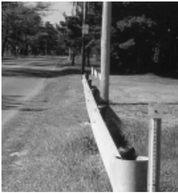
Beam guardrail will deflect several feet before it restrains a vehicle. This installation is dangerous. Also, there does not appear to be a good reason to install guardrail at this location.
