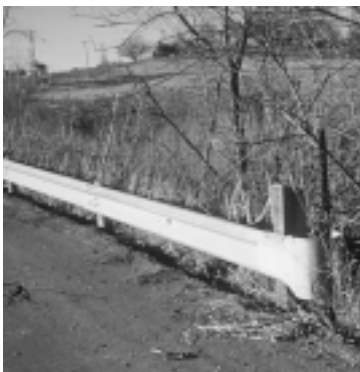
This rail is too low and could cause a vehicle to roll over. A minimum height of 27 in. to the top of the rail is recommended. Also, the blunt end can be hazardous. In addition, the intermediate posts are missing. Posts should be spaced at six feet three inches apart. Upgrading the guardrail is desirable if it is to be effective.
