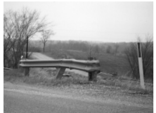
Short portions of rail are not as effective or able to restrain a large vehicle as longer ones. The guardrail in the bottom photo seems to be needed. Both need repair and are a hazard in their current conditions.
