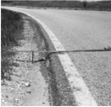
This drop-off is over five inches deep and is a hazard. Drop-offs commonly occur along the inside of curves and at intersections.
