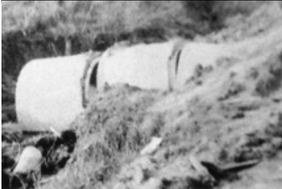
Water running outside a culvert washed away soil, weakening support for the culvert and the road.
