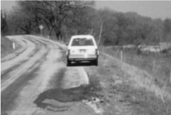
The road has been patched, but the real problem is a failing culvert.
