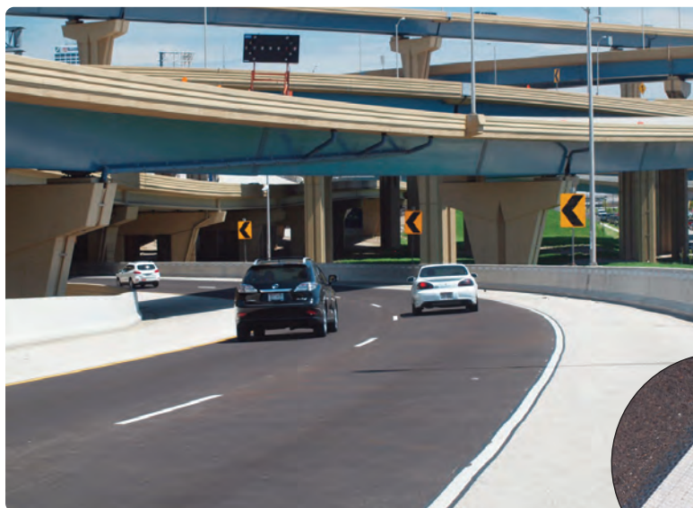
This ramp on the Marquette Interchange in Milwaukee averaged about 79 crashes annually, many during wet weather. The first full year after application of a high friction surface treatment, crash numbers dropped dramatically. INSET: HFST extends to the shoulder of the road.
