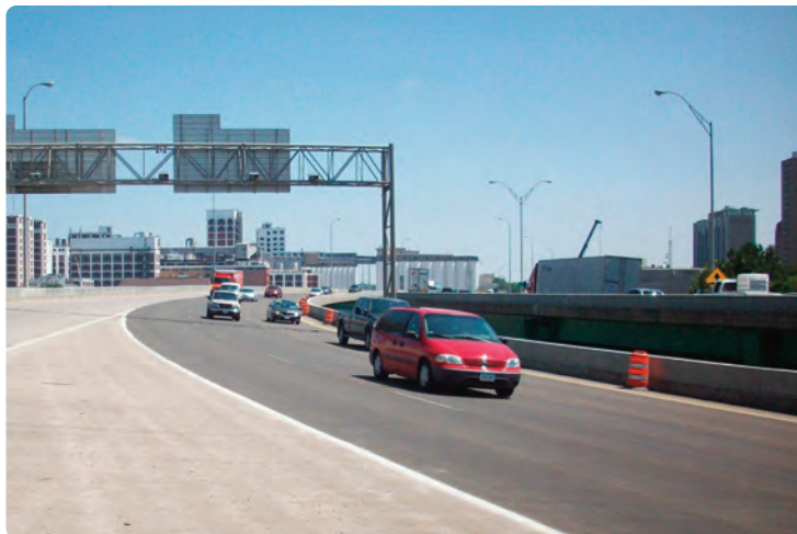
Two years after installation of HFST, the Cedar Rapids bridge deck shows no signs of deterioration.
