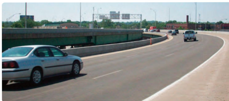
The contractors treated all three travel lanes of the Cedar Rapids highway bridge with an epoxy-aggregate to increase surface friction.
