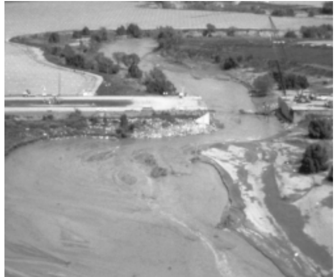
Scour is the suspected cause of a March 1995 bridge collapse on I-5 in California. Seven people died.
