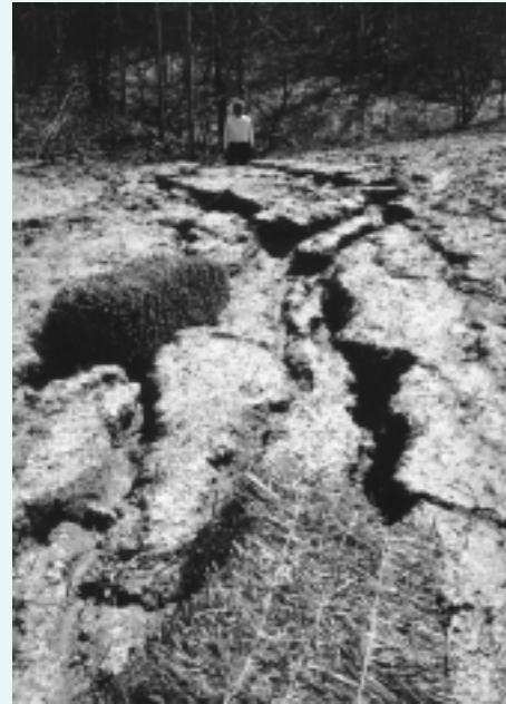
Too little, too late. Plan ahead for erosion control. Have all materials on site before you make the first soil cut. FDM Chapter 10 can tell you how (see Resources pg. 6)
