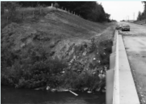
This small ditching project dumped tons of sediment into the river because no erosion control was used. Simple tools like matting, silt fences, hay bales, and rock riprap would have helped protect the river's water quality.
