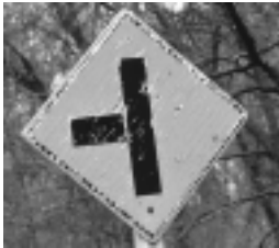
Poor condition signs are hard to see, especially at night, and should be replaced promptly.
