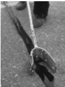
Cracks must be at least 1/4" for sealant to work.
