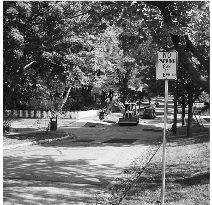
Working in the right of way without proper signing is a hazard that occurs frequently.
