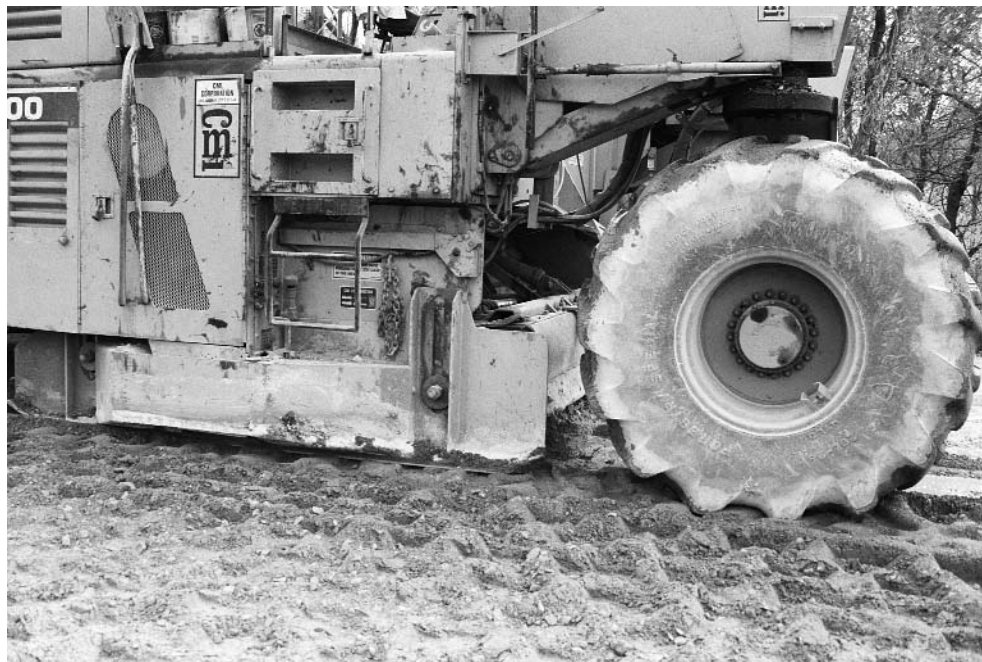
Pulverizing old pavement with base and subsoil provides strong support for a new asphalt layer.
