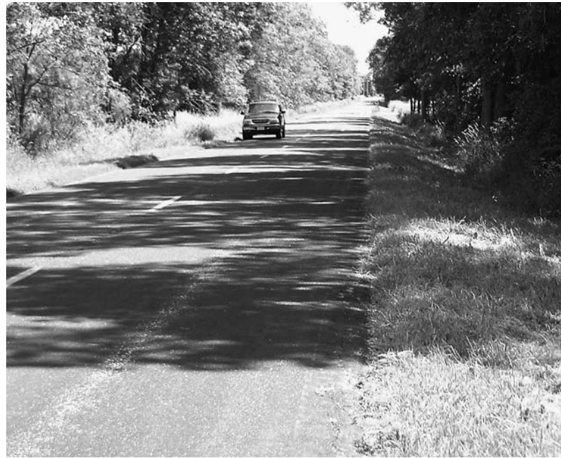
Daylighting a road by cutting down trees that shade the pavement reduces winter maintenance and gets damaging ice off the road surface.
