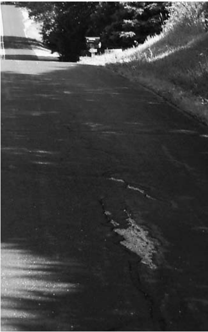
Pavement damage caused by ice in shaded area.
