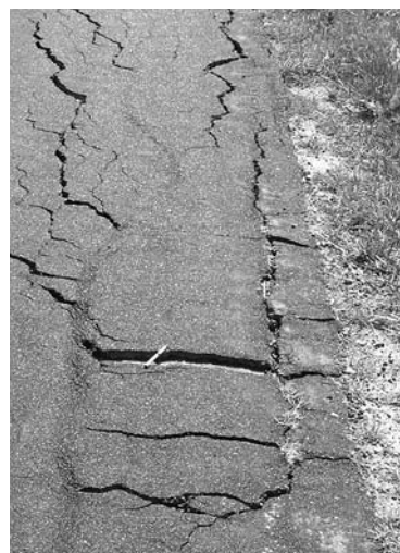
Pavement edges deteriorate when a road lacks shoulders.
