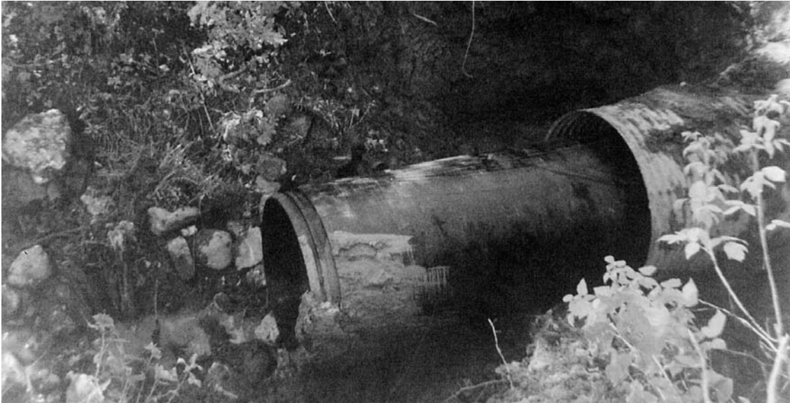
Sliplining with plastic pipe left deep fill in place, and the crew finished in one day.
