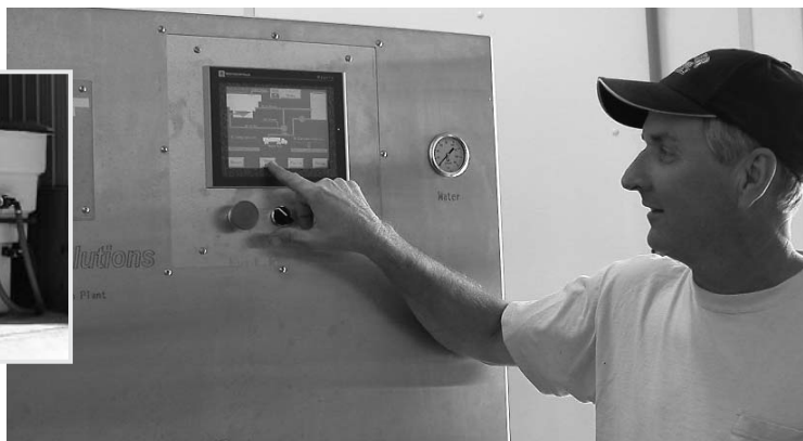
Gary Keegan uses touch-screen controls to program salinity and view the progress of the run. INSET The large 2.5-yard mixing bin is mounted in an enclosure adjacent to computer controls.
