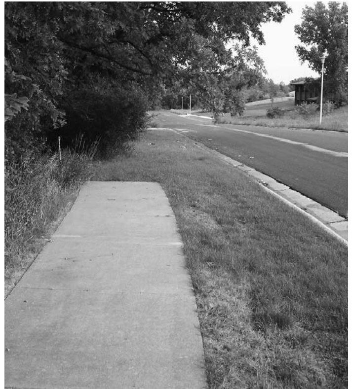
AT LEFT AND ABOVE: Sidewalk gaps and defects gain or lose maintenance priority based on local government policies.
