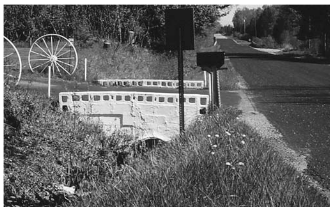
Driveway headwall close to the road presents a risk to motorists and liability for local governments.
