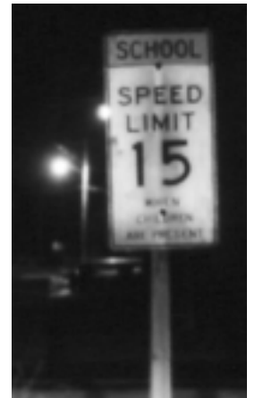
Night inspections are crucial. This sign which seems fine in daylight, is barely visible at night. White measured 4.5 candlepower, yellow 2; the minimum is 35.
