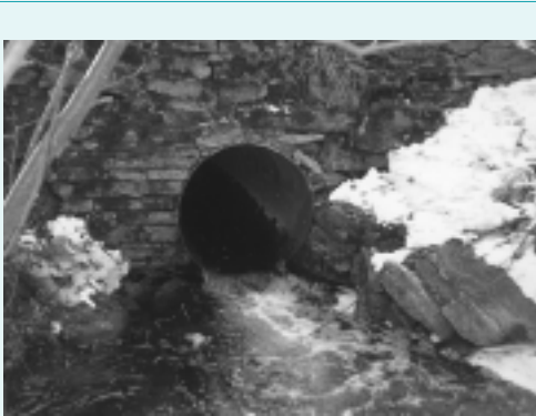
This culvert was set too high. Brook trout cannot pass through it to spawning areas on this Class I trout stream.
