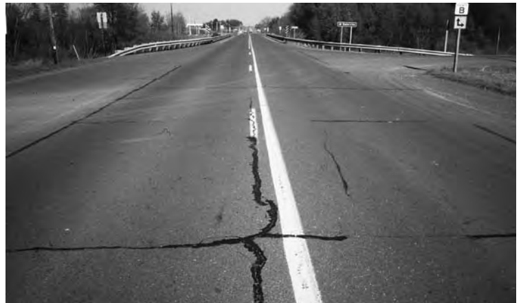
Getting the most out of WISLR starts with creating a current record of pavement conditions. This road rates a 7 on the PASER scale, indicating that routine maintenance will extend its useful life.
