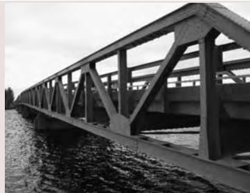
The six-span steel truss CTH M Bridge over the Chippewa River has a new load rating and posting BELOW after a review in 2007.
