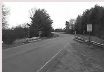
The CTH J Bridge in Lincoln County, LEFT due for replacement next year, has an updated posting after the 2007 review, as does the Axen Road Bridge, RIGHT which remains in good shape.
