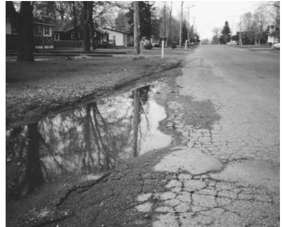
Poor ditch and shoulder drainage cause pavement damage.
