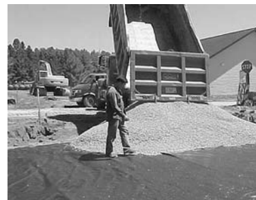
TOP: Careful installation of geotextile is important. БОТТОМ: Fabric holds clay back, keeping it out of the aggregate.
