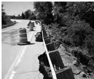
Drums warn motorists of a washed-out road.
