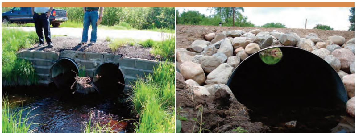
These photographs illustrate projects where the DNR will work with local governments to improve roads and culverts under the new general permit. The deteriorating culvert at left is a barrier to fish while the replacement on the right creates a good waterway passage.
