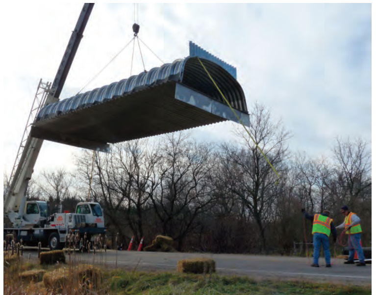
TOP: Local crews remove the old bridge deck and one abutment at the start of the one-week project. CENTER: Crews assemble the culvert on site. No individual piece was bigger than 4' by 6' and all weighed less than 100 lbs. BOTTOM: A crane lifts the new box culvert into place.
