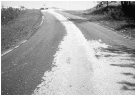
Roads like this rate 5 on PASER's 10-point scale: good structure but needing sealcoat or overlay.
