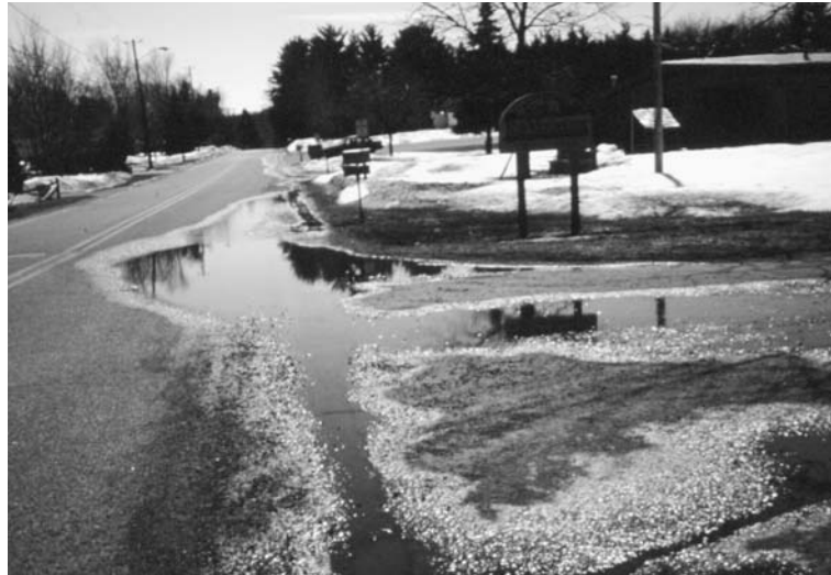
Drainage from an improperly constructed driveway can cause road damage.
