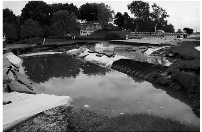
An example of serious damage to road infrastructure from Wisconsin's storms of summer 2008.
