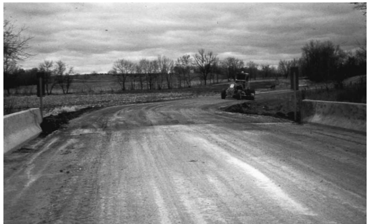
Grade bridge approaches to eliminate potholes and provide a smooth ride on to deck.
