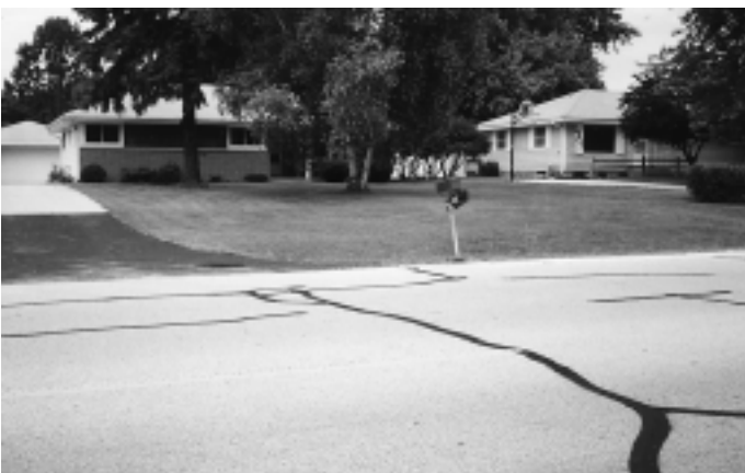
Crack sealing became a bigger part of Brown Deer's streets budget after PASER showed how it saves money in the long run.
