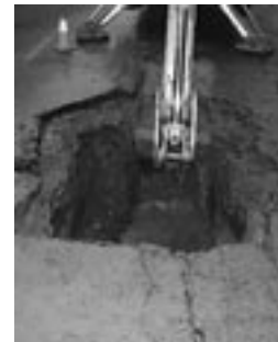
Jagged backhoe openings damage pavements.
