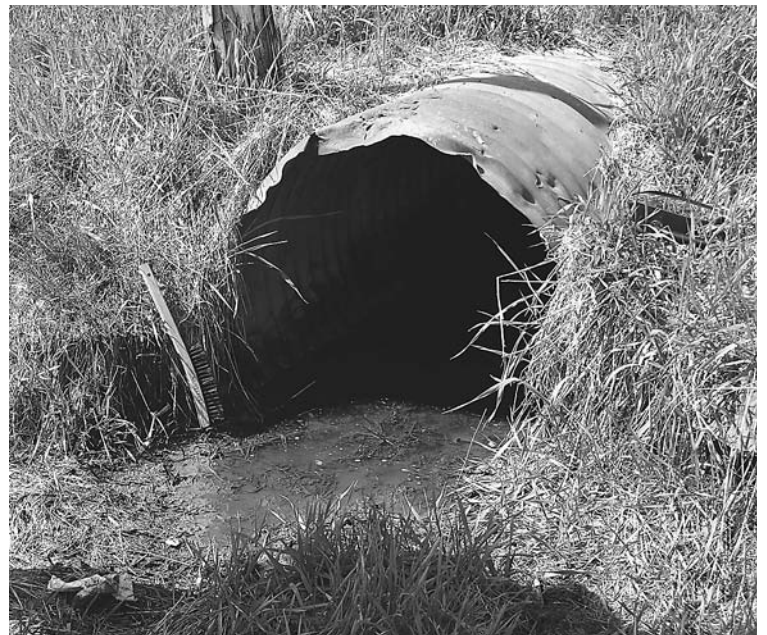
Poor installation left this culvert lower than the ditches. Constant standing water quickly rusted through the bottom.
