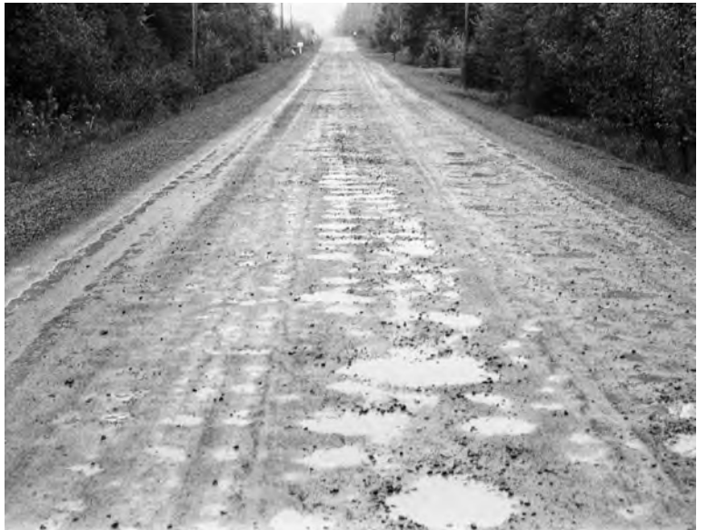
Careful design and regular maintenance prevents problems on gravel roads like washboarding ABOVE and severe potholes BELOW .
