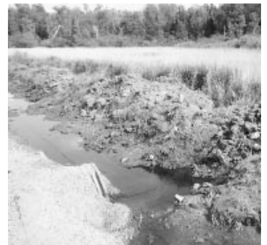
Side-casting ditch spoils into wetlands, as shown in these photos, is regulated by DNR.
