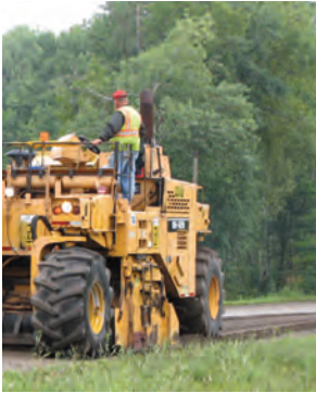
Pulverizing and blending the existing asphalt with a portion of new base aggregate.
