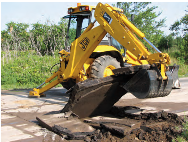
Many layers of old asphalt are visible during a saw-cutting operation to replace a culvert at the start of the road improvement project.
