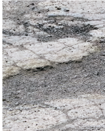
Rutting and cracks show poor condition of pavement before rebuilding.
