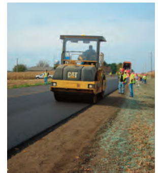
Crews roll the asphalt mat along the edge of the road on a Safety Edge installation.
