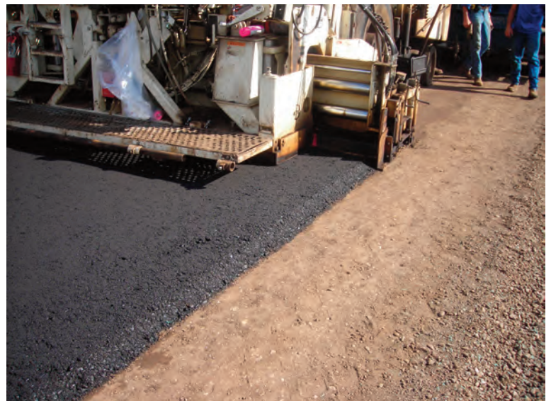
Paver places Safety Edge on Chippewa County Demonstration Day project last October.
