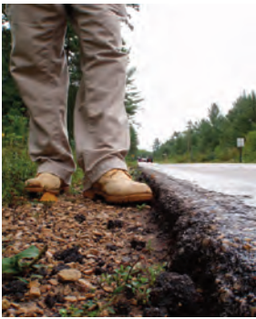
The Safety Edge detail replaces vertical edge drops like this with a sloped edge that helps drivers recover control after leaving the roadway.
