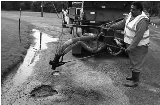
Spray injection patching works well under adverse conditions and produces long-lasting temporary patches.
