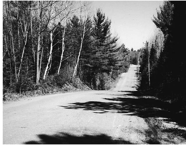
BEFORE Crass Road has many steep hills with very dangerous slopes, no drainage, and no place for snow removal.
