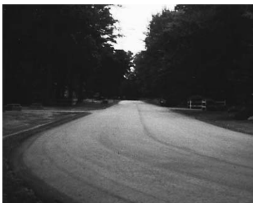
AFTER Now 22 ft wide, it has a new drainage ditch and improved curve. The town repaired lawns after the trees were cleared.
