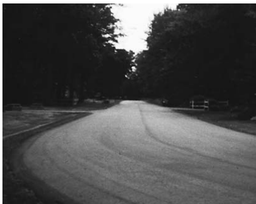
AFTER Now 22 ft wide, it has a new drainage ditch and improved curve. The town repaired lawns after the trees were cleared.
