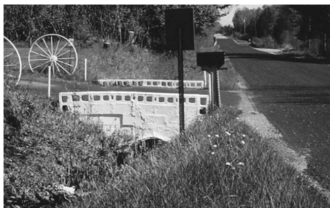
Driveway headwall close to the road presents a risk to motorists and liability for local governments.
