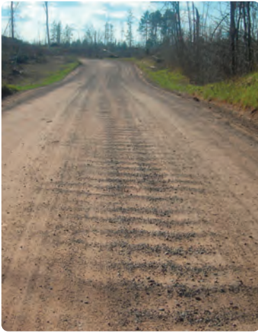
Traffic and loose gravel combine to create washboarding. A good aggregate mix can help prevent a recurrence of this condition.
