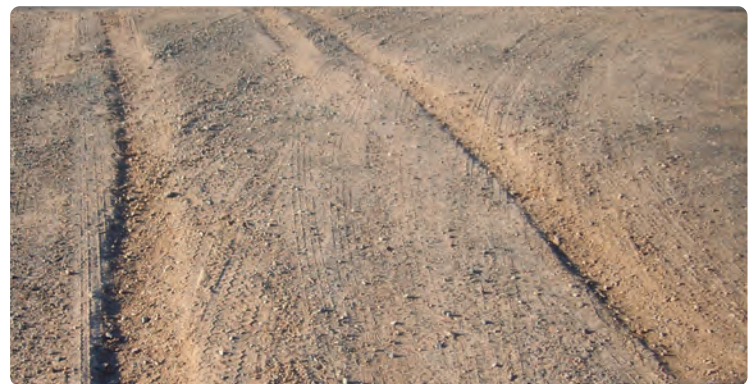
Severe rutting makes travel difficult and can require substantial repairs. Preventing this level of deterioration is important to gravel road maintenance.
