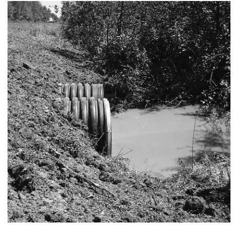
Culvert installed without erosion control measures quickly affects water quality.
