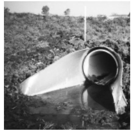
Plastic liners have higher flow rates than corrugated metal. Grout fills the cavity between liner and culvert.
