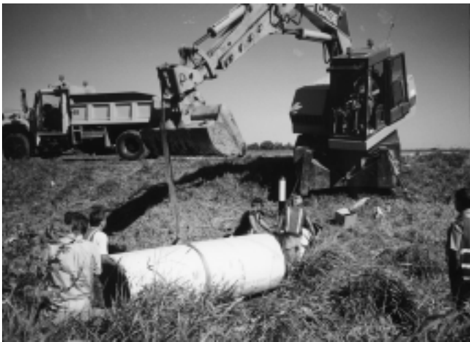
Plastic liners are an economical alternative to culvert replacement.
