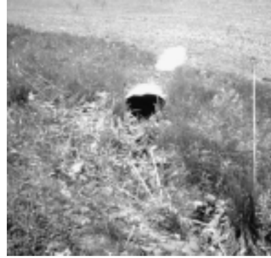
Culverts need proper cover and end treatments to prevent erosion and undercutting.
